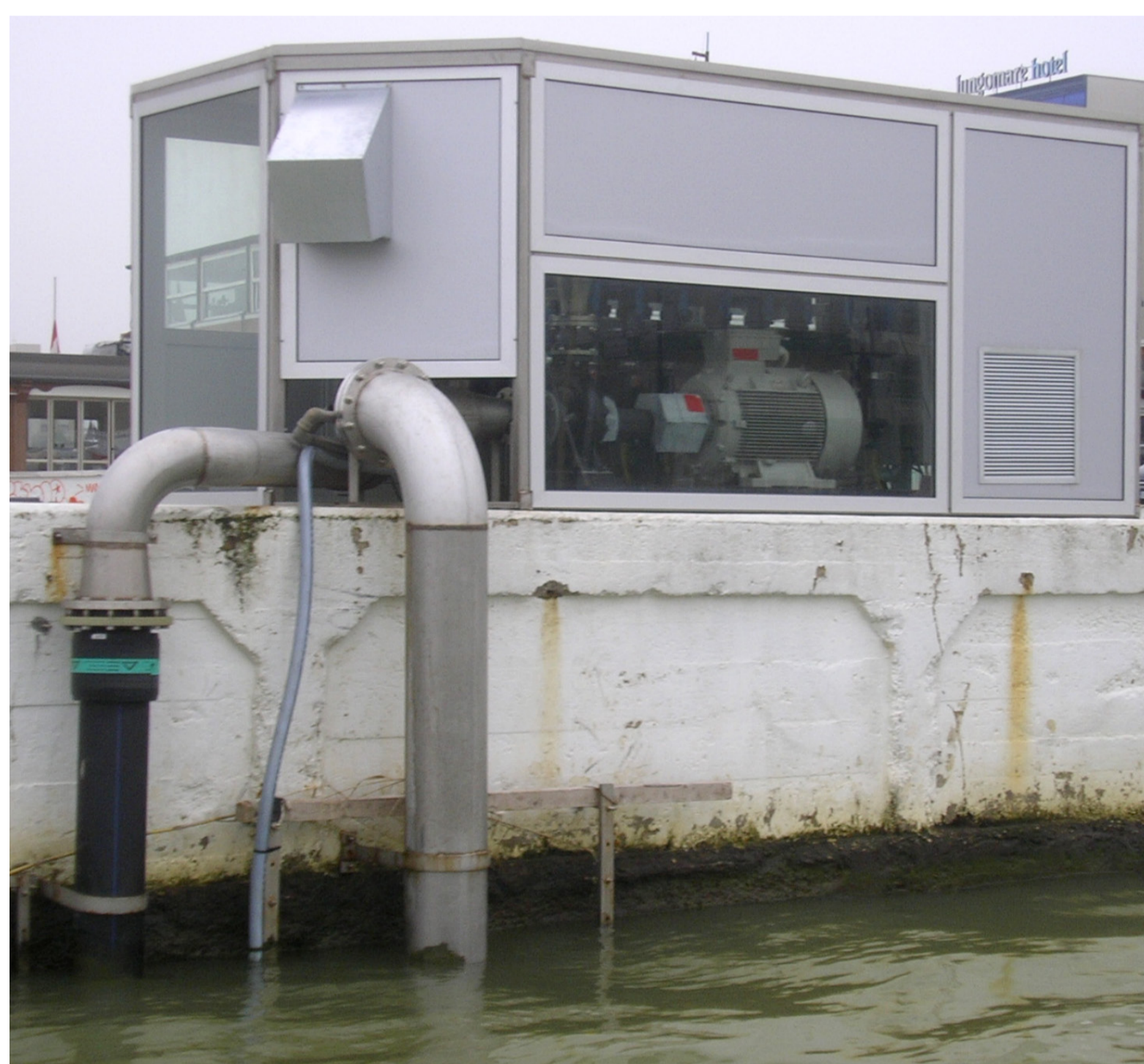
Portoverde pumping station
